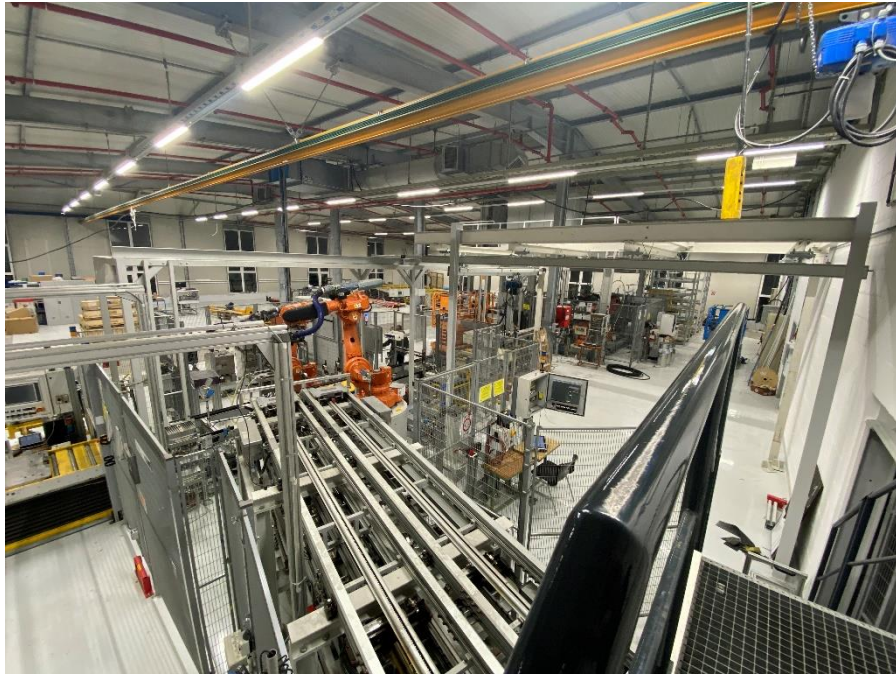
View on the Battery Pack assembly line
